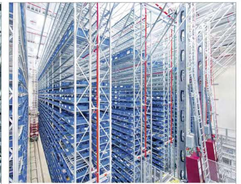
Automatic Storage and Retrieval System
