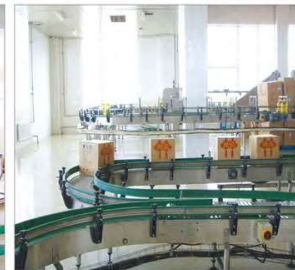
Finished carton conveyor
