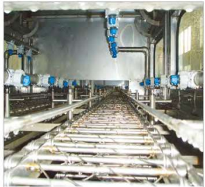
High pressure cleaning spray room interior
