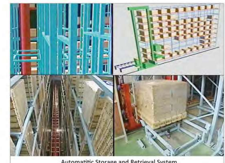
Automatic Storage and Retrieval System
